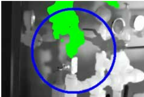
Quantifies gas, such as the methane escaping this wellhead valve at 0.59 lb/hr
